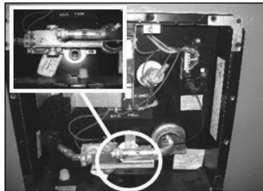
Fig 1: Water Heater Drain Plug
