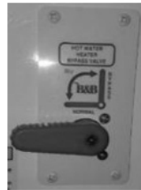
Water Heater Bypass
