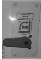
Water Heater Bypass
