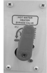
Water Heater Bypass
