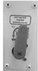
Water Heater Bypass
